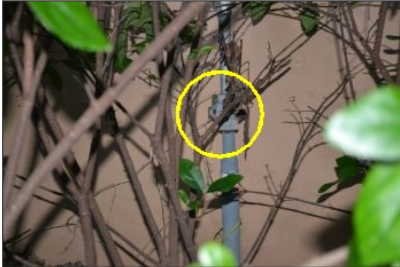
Main gas shut off valve was located at the right side of the home exterior
