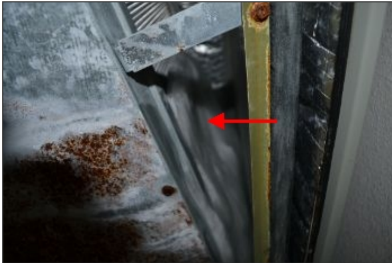
Unit #2 (Ice noted)
