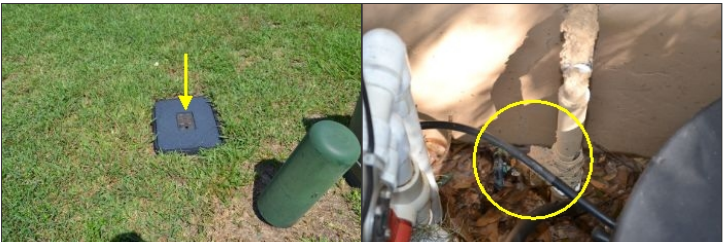
Water meter was located at the front yard of the home.
